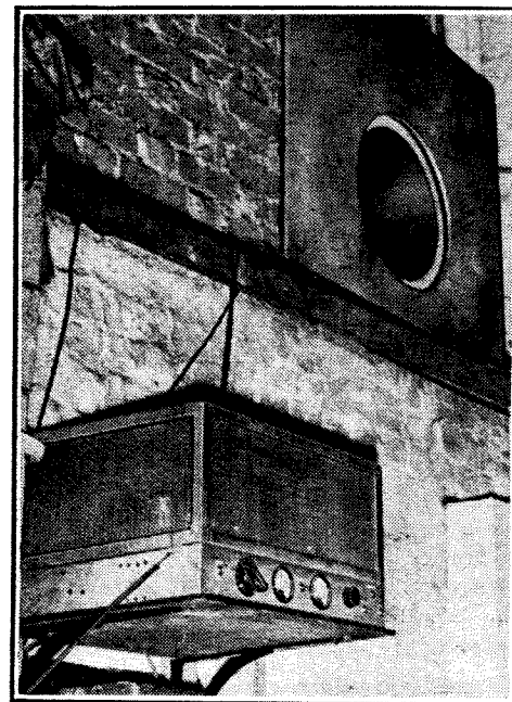
Back-stage speaker at the Adelphi. One of the associated amplifiers is mounted on brackets on the wall.
